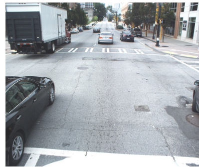
Fig. 6. Camera image of cracked pavement
